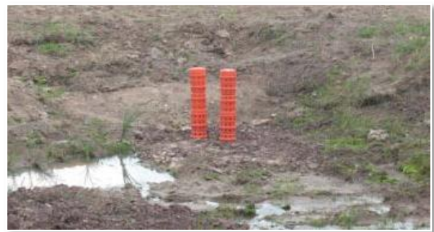
Figure 3. Surface water inlets.
